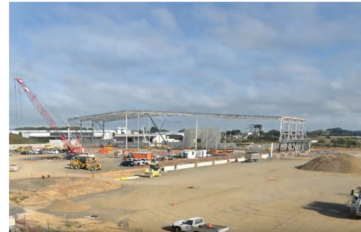
Foodstuffs North Island's new chilled and frozen distribution centre is set to open in 2028
